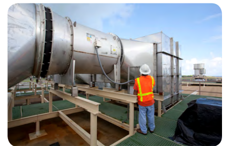
Paint Booth Exhaust
