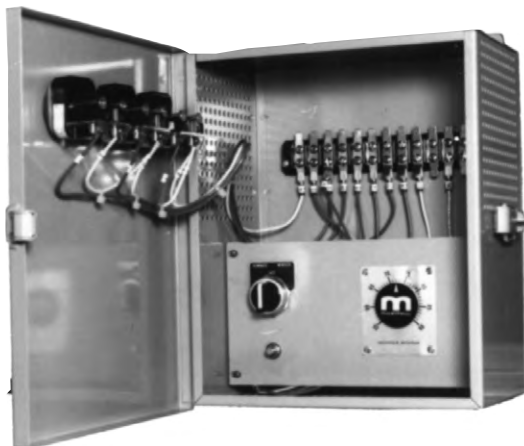
Outlet Temperature Control (OTC)
